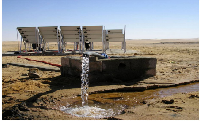
Figure.20. PV Water Pumping Beer Tssawa
