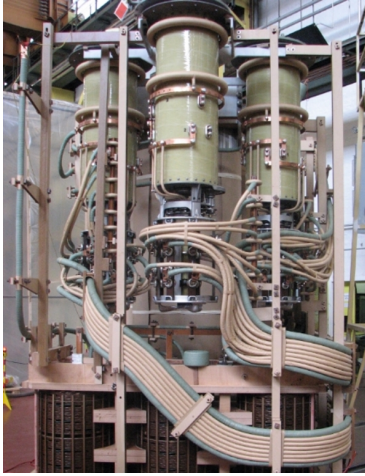
Figure 1: Power transformer with a regulation unit
