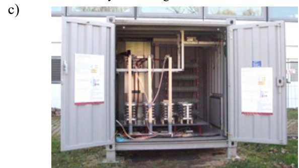
Figure 5. 3D CAD model (a), photo of the power electronic grid excitation circuit (b) and photo of the medium-voltage measurement container
